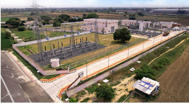
220 KV Sub - Station
